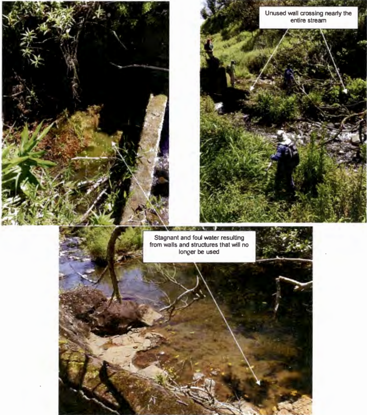
Figure 8. East Wailuanui at Koolau ditch (K-18). Stagnant water outside the west wall (top left), wall crossing stream (top right), stagnant water on the east side of the stream.
