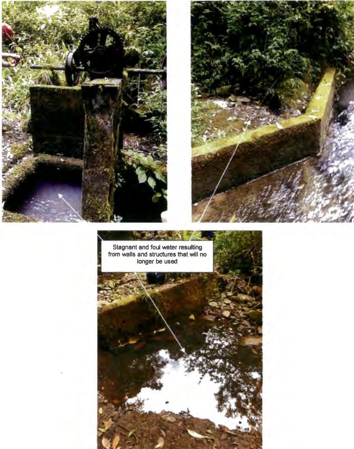
Figure 4. Stagnant water standing in depressions created by the walls and the gate structure.
